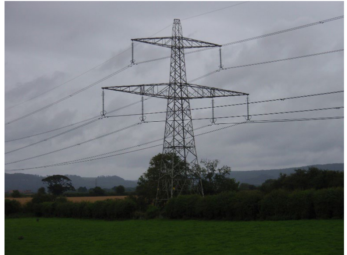
Image 1.2 Typical suspension low height lattice pylon
