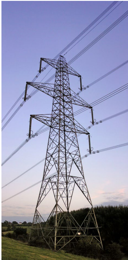
Image 1.1: Typical suspension 'traditional' lattice pylon
