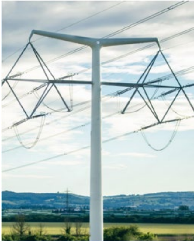
Image 2.2 Typical tension T-pylon
